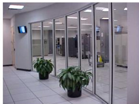
Racks are environmentally secured
